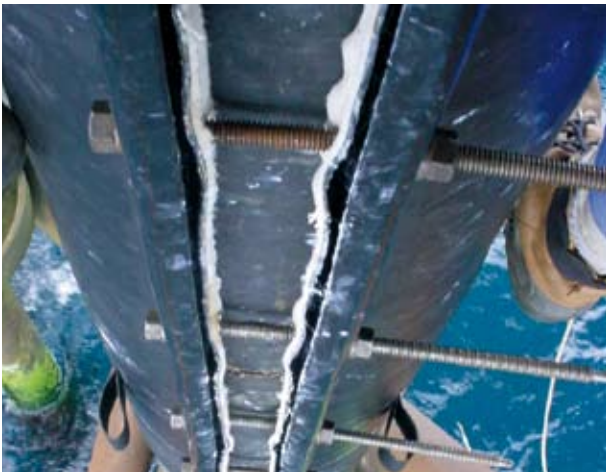
Rope access installation of Retrowrap HD in multiple 3m lengths being tensioned by reusable draw bolts prior to fitting permanent bolt sets.
