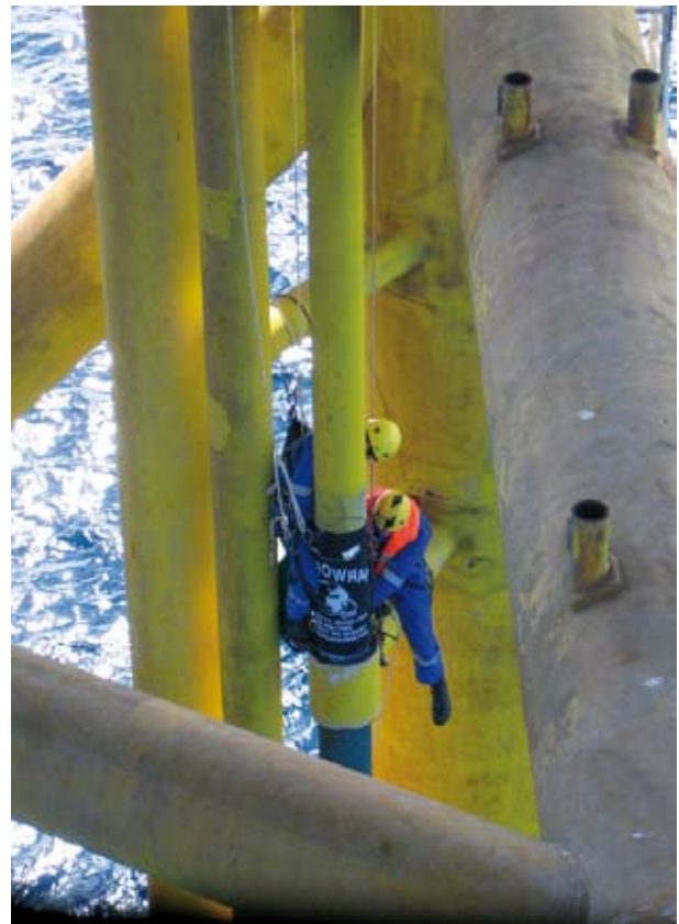
Rope access team installing dual diameter Retrowrap above riser clamp after cutting back disbanded neoprene.
