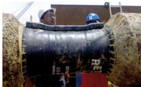
Laywrap PQT of subsea replacement field joint coating Arabian Gulf. Note thermally formed flanges follow joint contour. prior to fitting permanent bolt sets.
