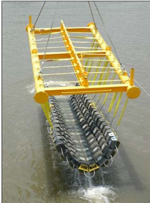
This CP Mat™ is being deployed as a primary retrofit for a damaged pipeline.
