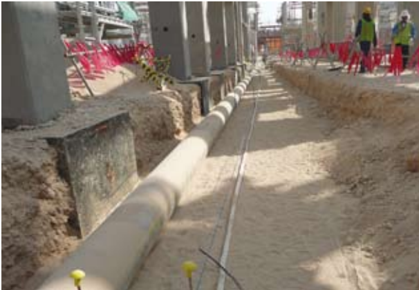
MMO Linear Anode alongside pipeline
